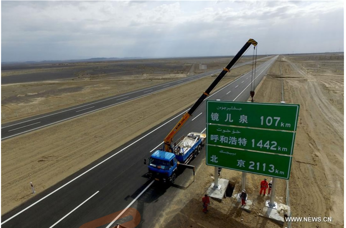
Workers set up a traffic sign at the Hami section of Beijing-Xinjiang expressway in Hami, northwest China's Xinjiang Uygur Autonomous Region on June 18, 2017. /Xinhua Photo
