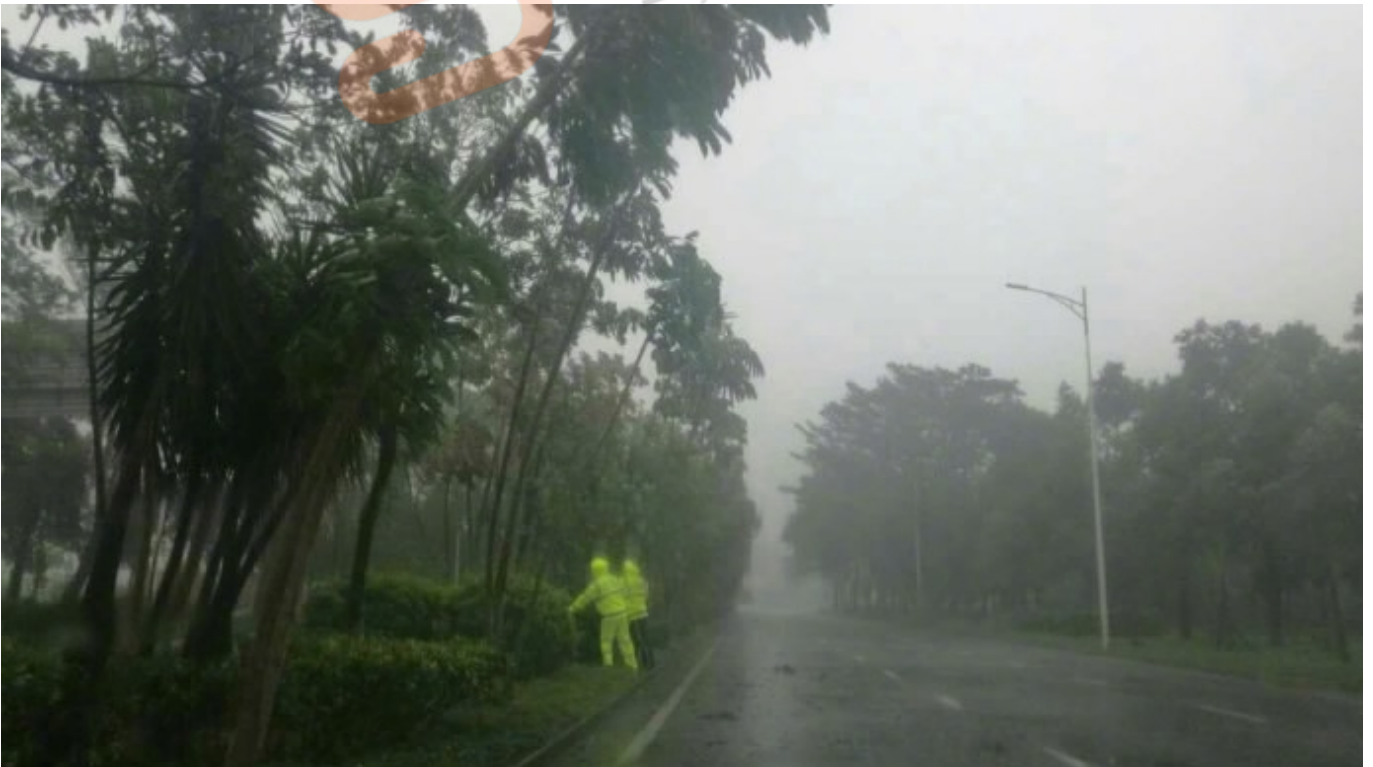
Cleanup work is underway in Shenzhen, south China's Guangdong Province on August 27, 2017. /Weibo Photo
